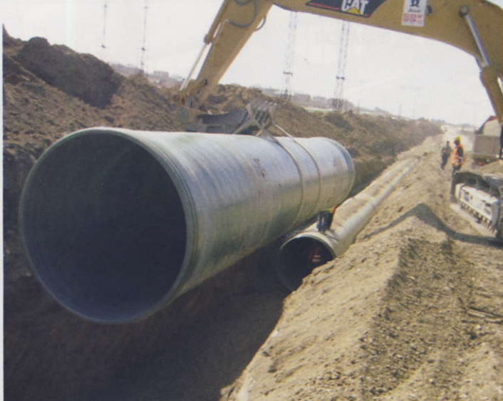
The low weight of the GRP pipe reduces the size of the lifting equipment required, lowering installation costs.
