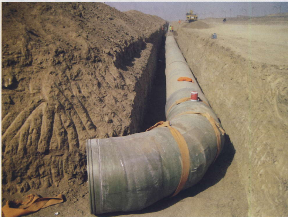
Each section of pipe is 12 m long and the pipeline will require 25 000 joints.
